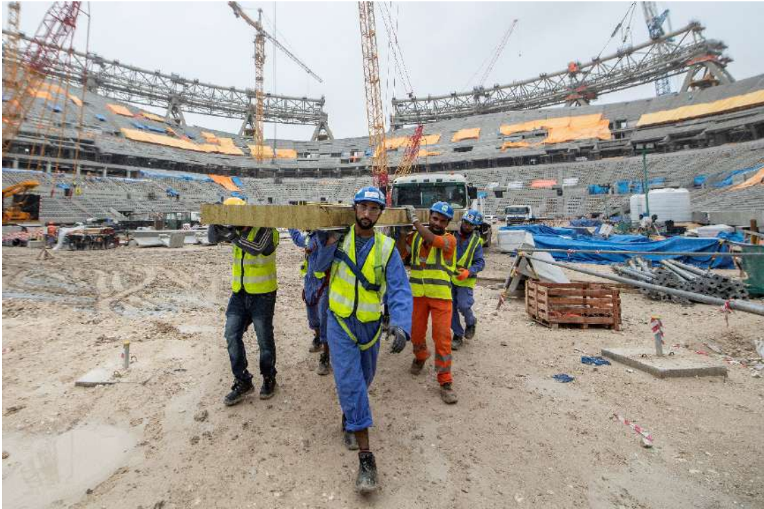
Migrant workers constructing the Lusail Stadium on December 10, 2019 in Doha, Qatar. The Lusail Stadium will host the opening match and the final match of the next FIFA World Cup Qatar 2022. © David Ramos - FIFA/FIFA via Getty Images
