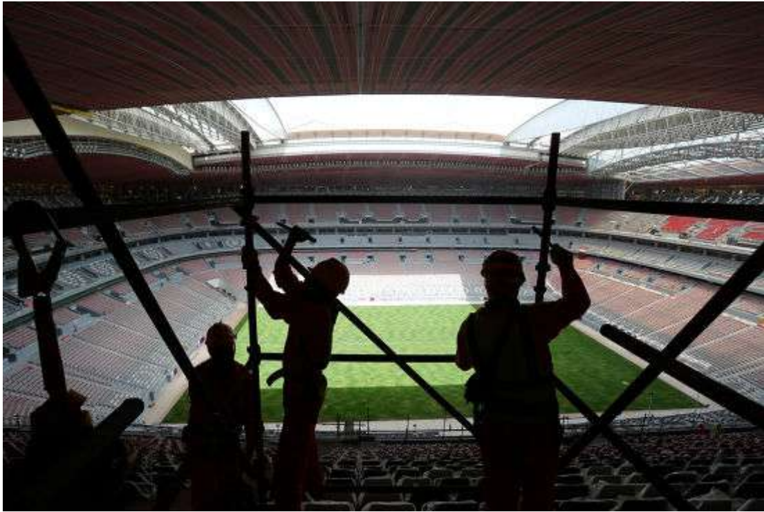
Workers remove scaffolding at the Al Bayt stadium in Al Khor, Qatar, about 50 kilometres (30 miles) north of Doha. © Kamran Jebreili/AP/Shutterstock
